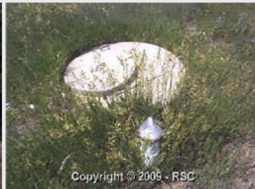
Well head & pit.
